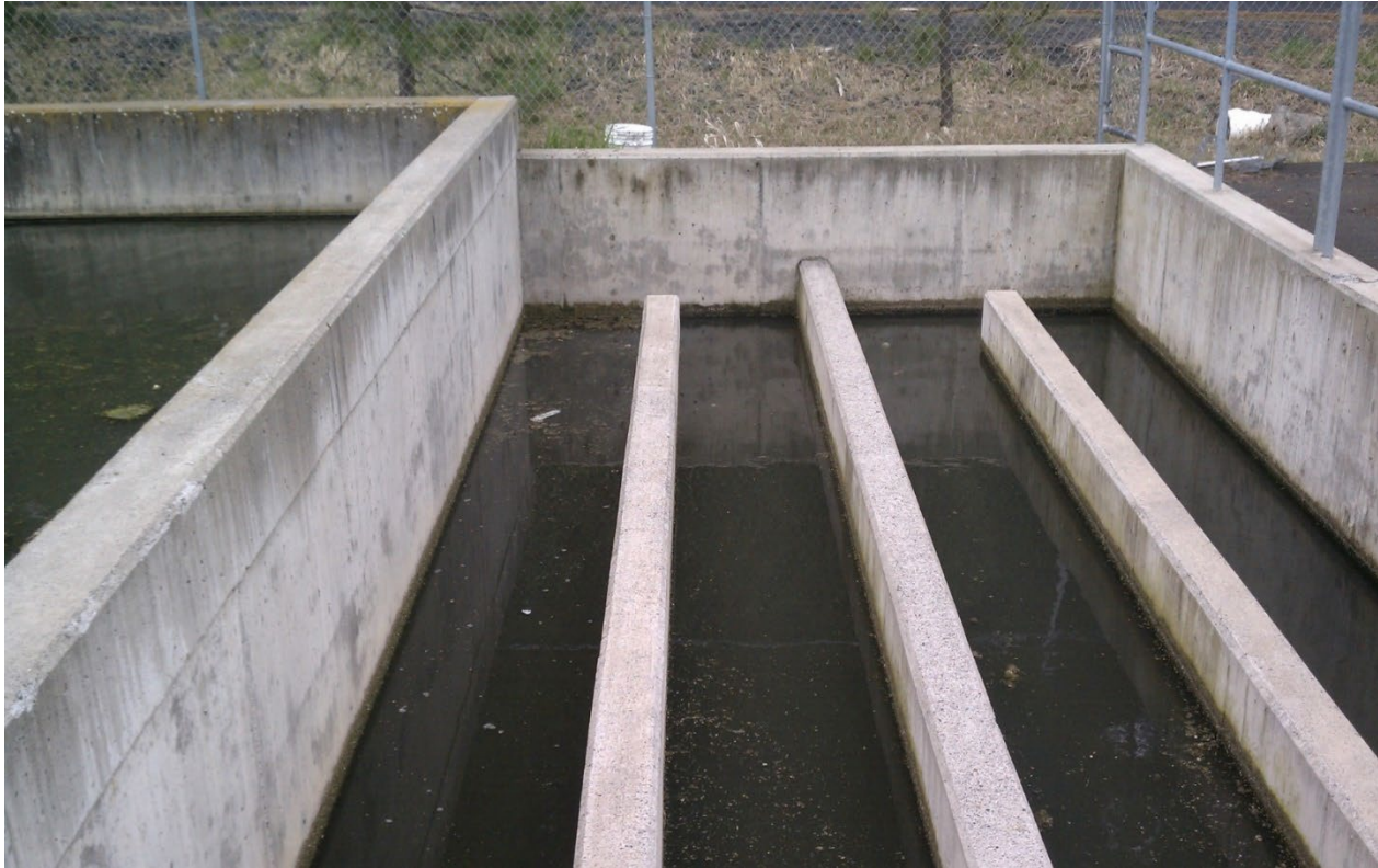
Photo 2-8: Chlorine Contact Basin
