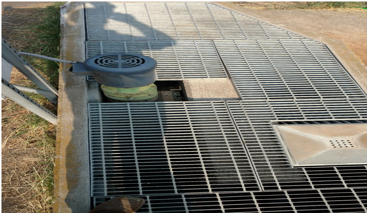
Photo 2-3: Pretreatment with Electric Comminutor and Manual Bar Rack
