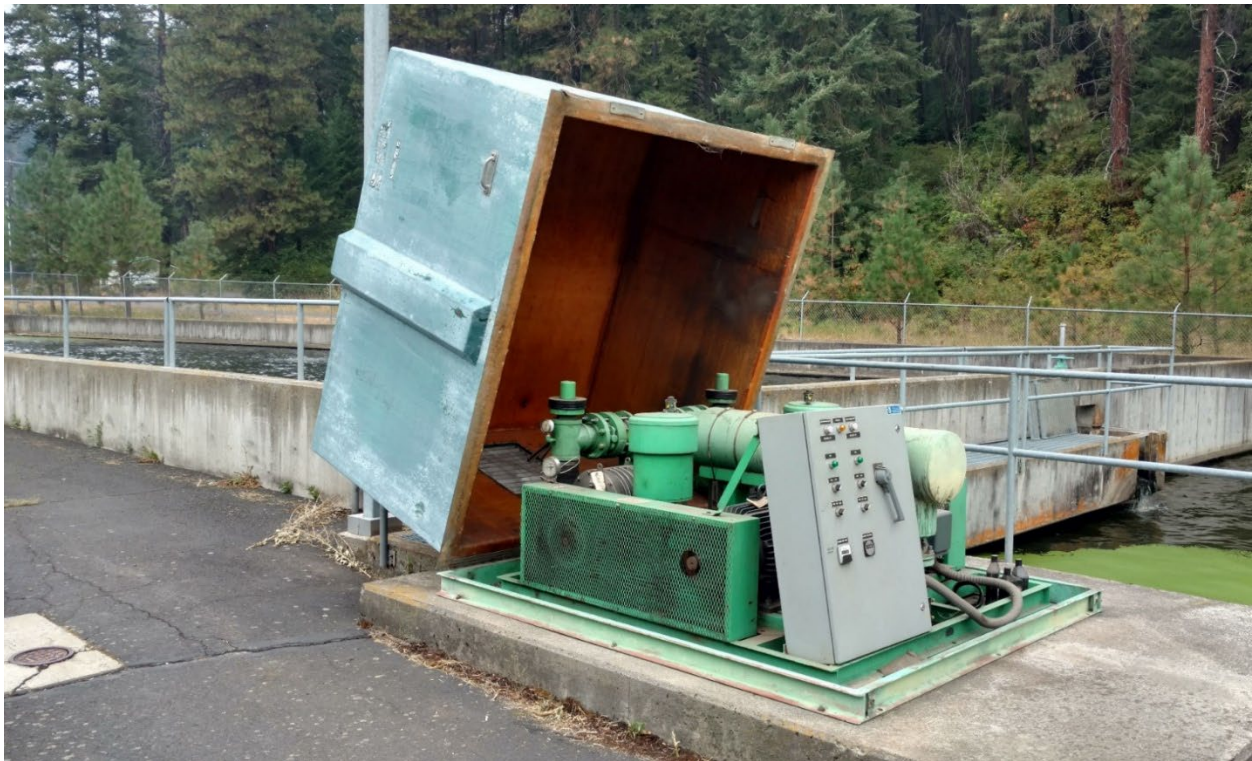
Photo 2-4: Aeration System Blowers
