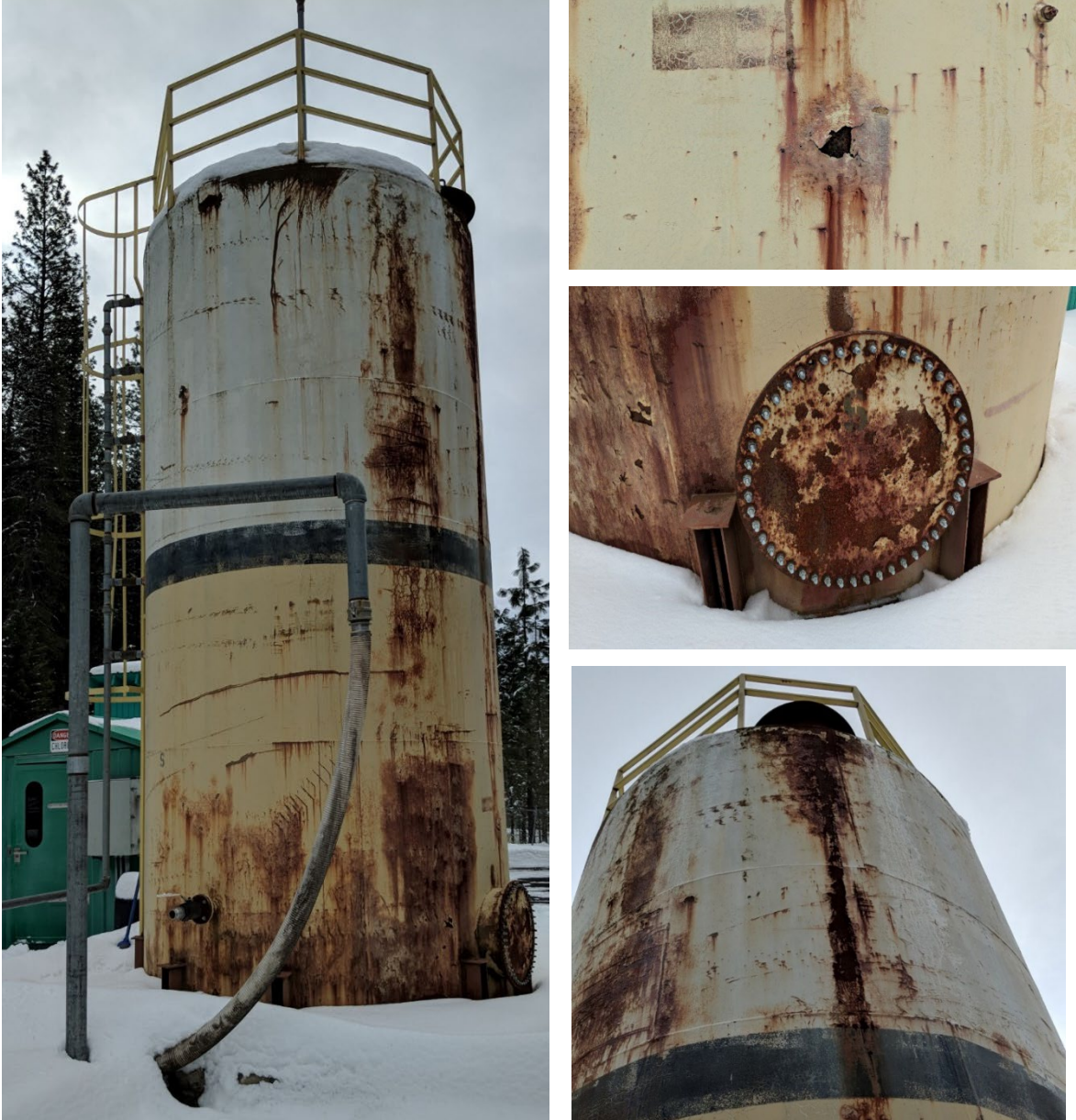
Photo 2-6: Aerated Sludge Holding Tank
